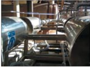
A Prosonitron system installed for processing in the alumina industry.
